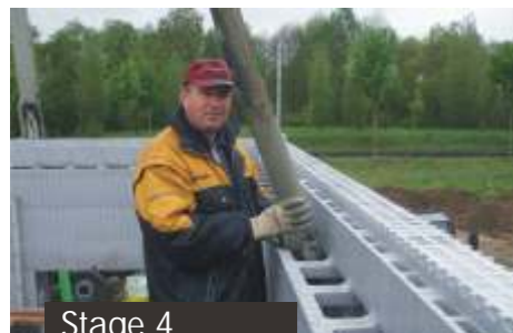
Stage 4 Concreting with a pump up to the height of one storey
